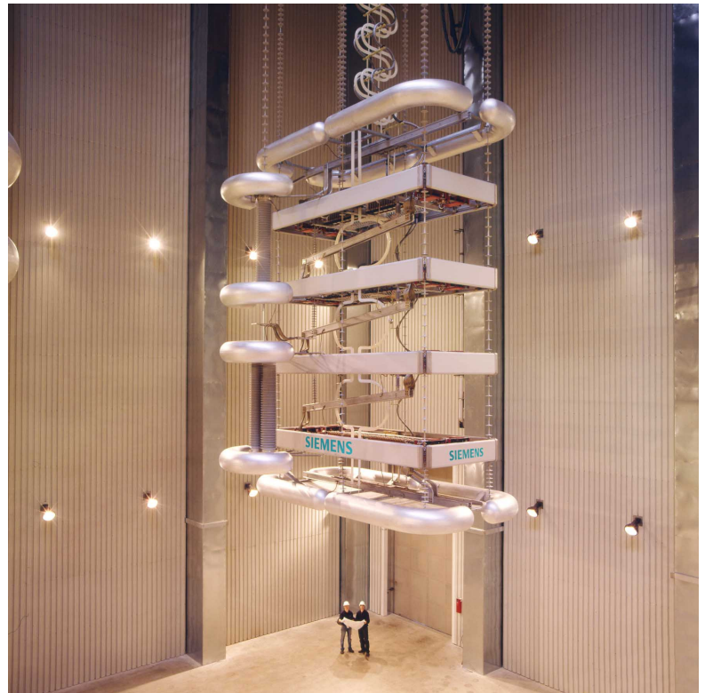
Fig. 2: Indoor photo of valve hall
