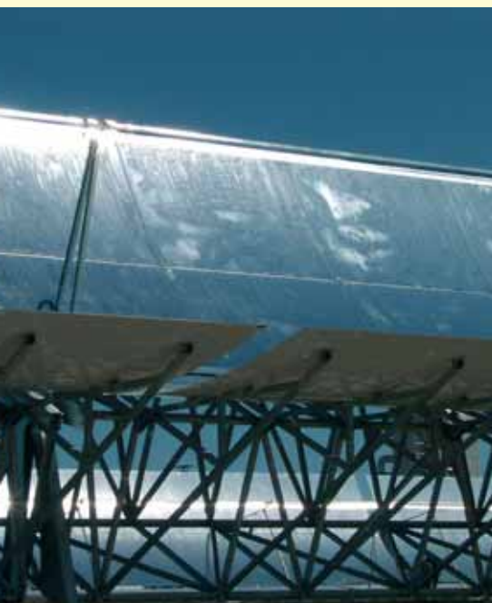
Enhanced parabolic trough structure of the EUROTOUGH project facility at Plataforma Solar de Almeria, Spain
