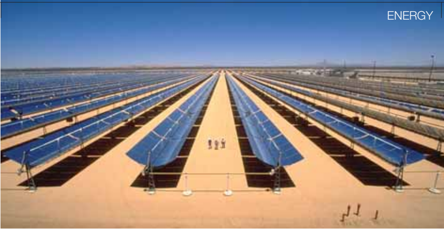
Figure 4 Parabolic trough concentrating solar collector field of the 150 MW (5 × 30 MW) steam cycle solar electricity generating systems at Kramer Junction, California (Source: KJC)
