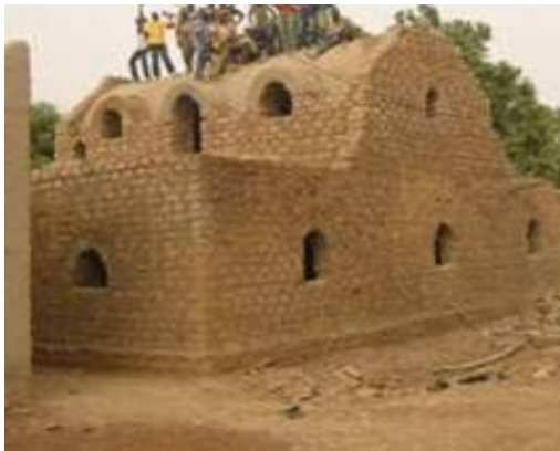
Fig. 8: Resilient earth building technology, Sahel - no-wood build, reducing deforestation, better thermal performance at 10% of normal construction cost. (Source: La Voûte Nubienne. http://www.lavoutenubienne.org/ )
