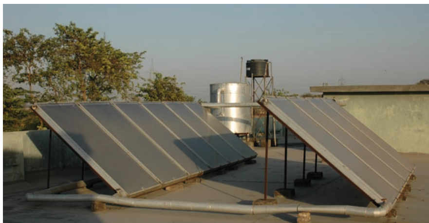
Rooftop solar water heaters are one of the most well known ways in which sunlight can be harnessed for residential applications.
